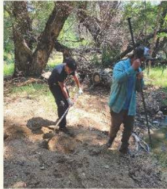
Figure 4: DeVaun and BLM staff digging a hole for a new fencing brace.
